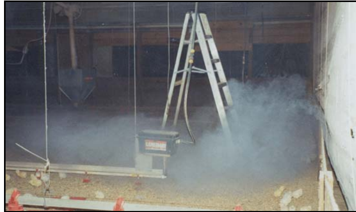
Figure 1. Smoke showing air leaking into brooding area.
